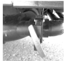
Grey Tank Drain
