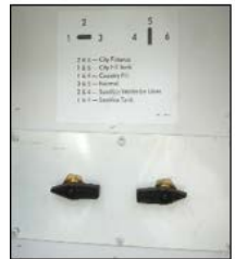
Fig. A - Water Valve Controls
