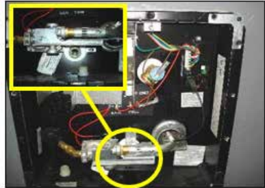
Fig 1: Water Heater Drain Plug
